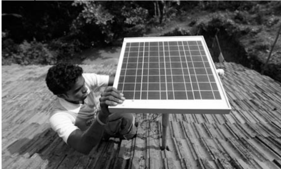
Sharan Pinto installs a solar panel on the rooftop of a house in Nada, a village near the southwest Indian port of Mangalore, India. Photograph: Rafiq Maqbool/AP
