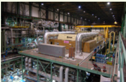
2011: Turbine hall with turbines © Javys.
