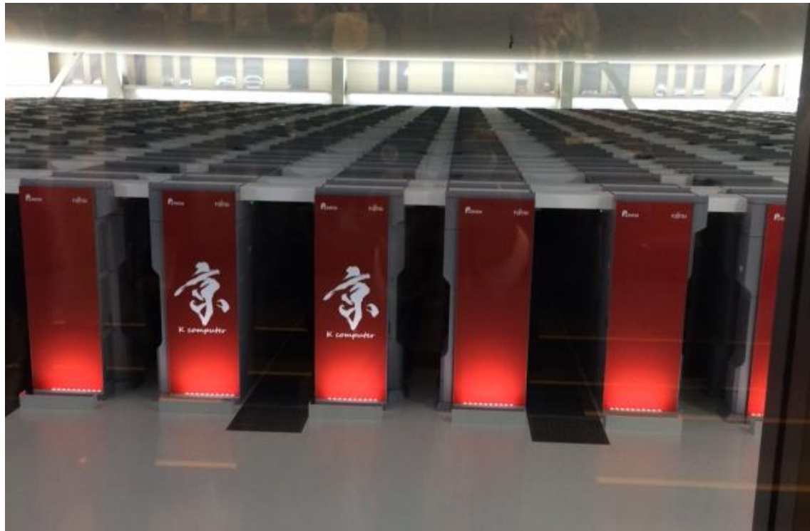
Big data storage facility in Japan
