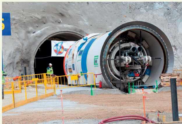
Photo 2 — Section of high voltage direct current interconnector cable being installed in the tunnel under the Pyrenees
