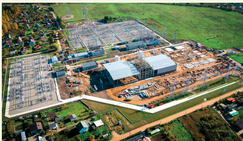
Photo 3 — NordBalt ground station in Klaipeda, Lithuania
